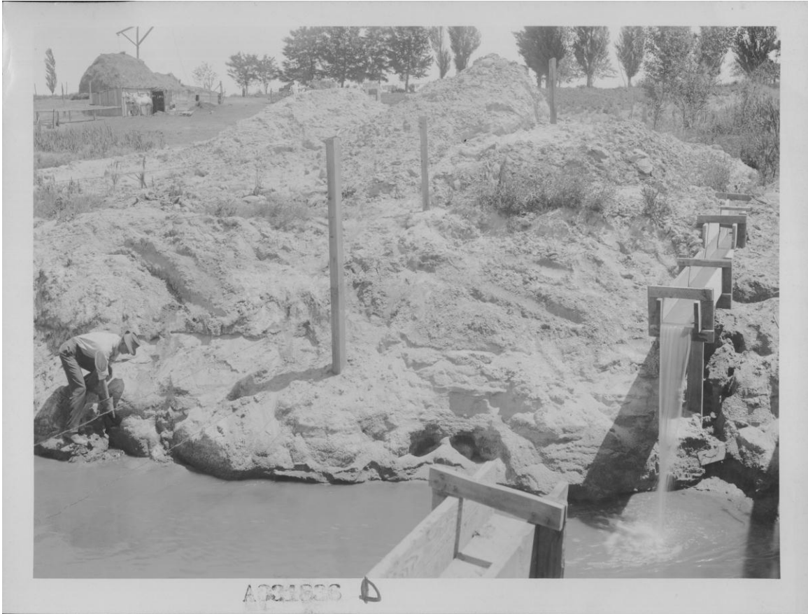
Figure 18 (no date, likely June 22, 1914) "View showing drainage from water bearing strata on Mason Creek Drain." 104
