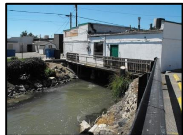
Above: Keystone Pizza is one of the last buildings remaining over Indian Creek.
